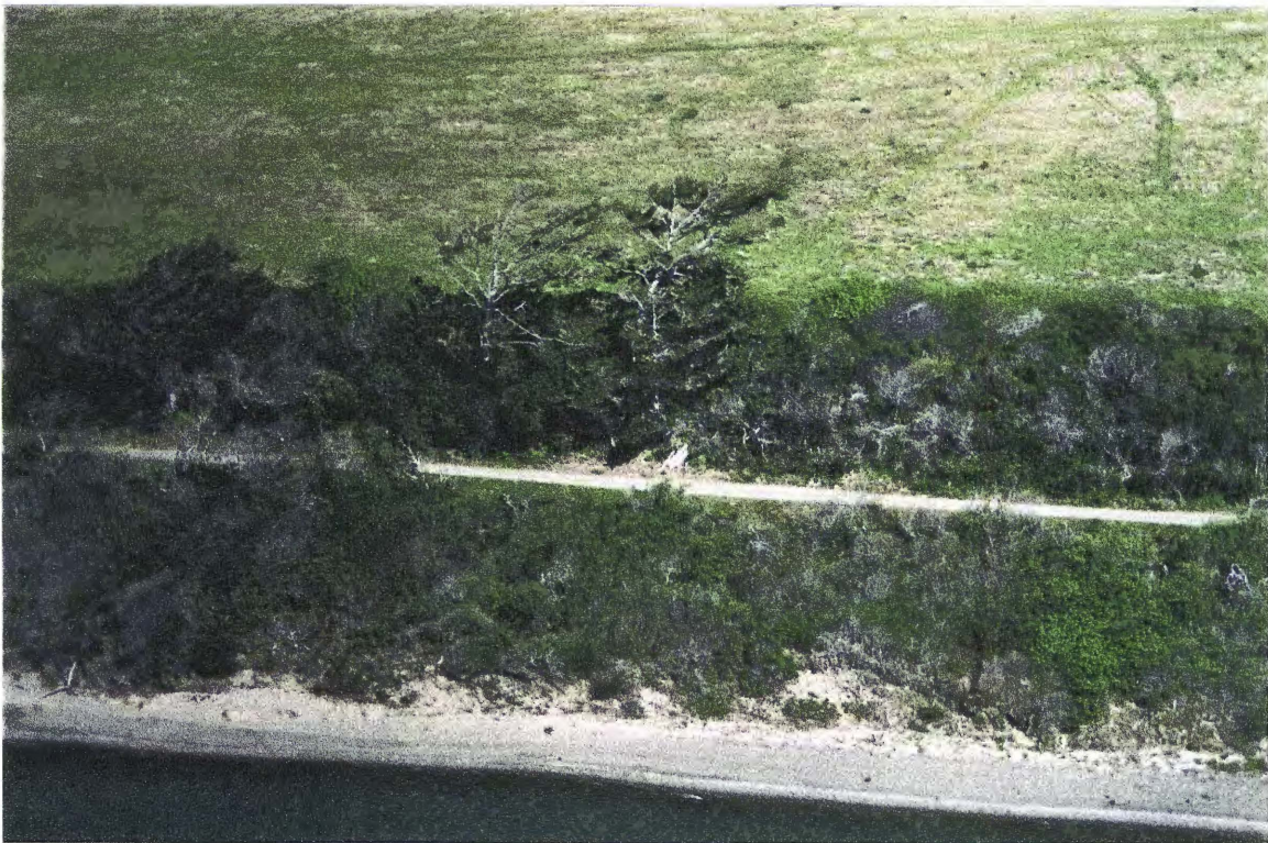
Erosion at Sand Pointe Subdivision site.
