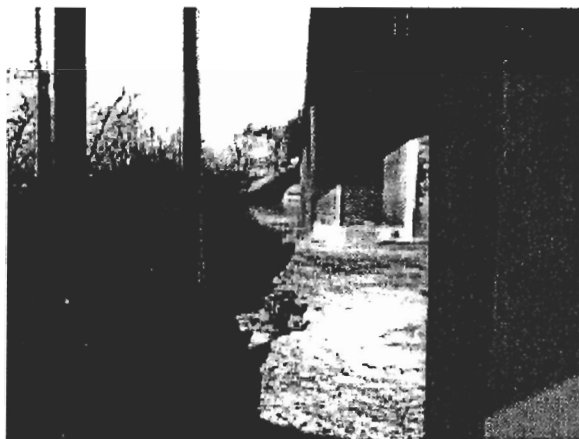
Photo 18. Drainage ditch southwest of the south side of the bridge (facing north).
