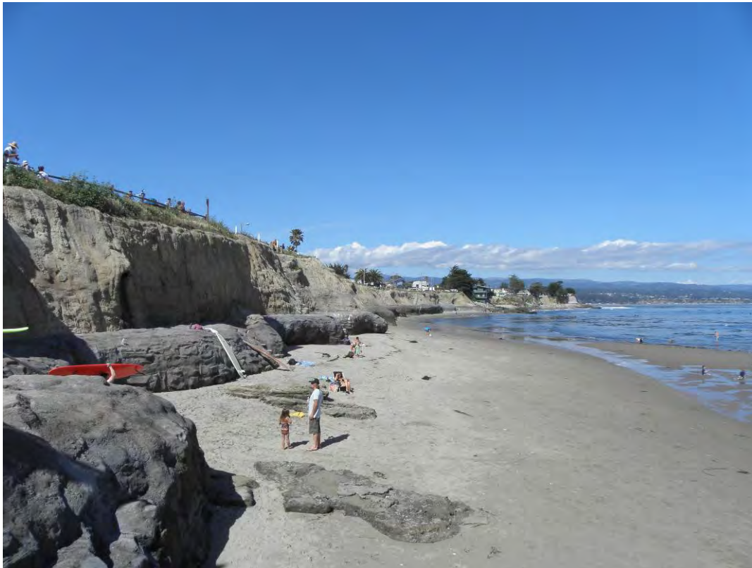
Figure 2: Photo of Seawall at Pleasure Point. Designed and built to blend with natural bluff conditions.
