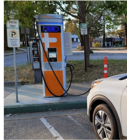
Level 3 charger (DCFC)
