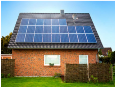
Residential roof-mounted solar
