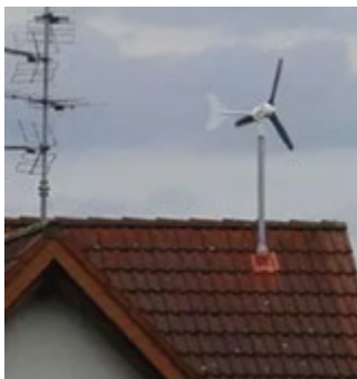
Roof-mounted wind turbine
