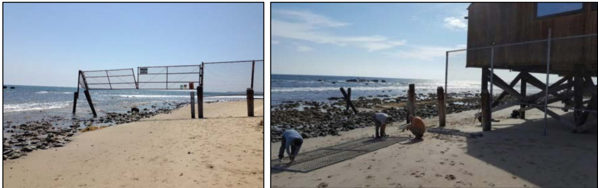
This illegal fence was removed from a Malibu Beach, in accordance with an agreement negotiated consistent with Section 30821.
