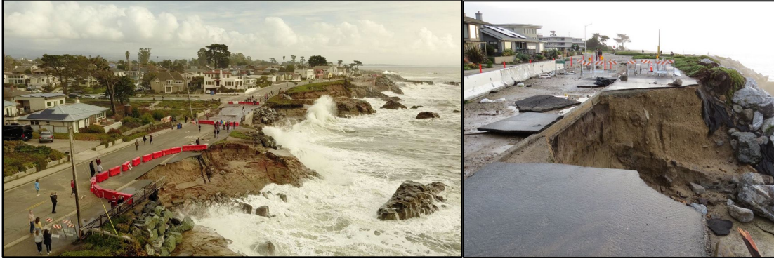
Damage to West Cliff Drive in Santa Cruz during high tides and extreme waves in January 2023.
