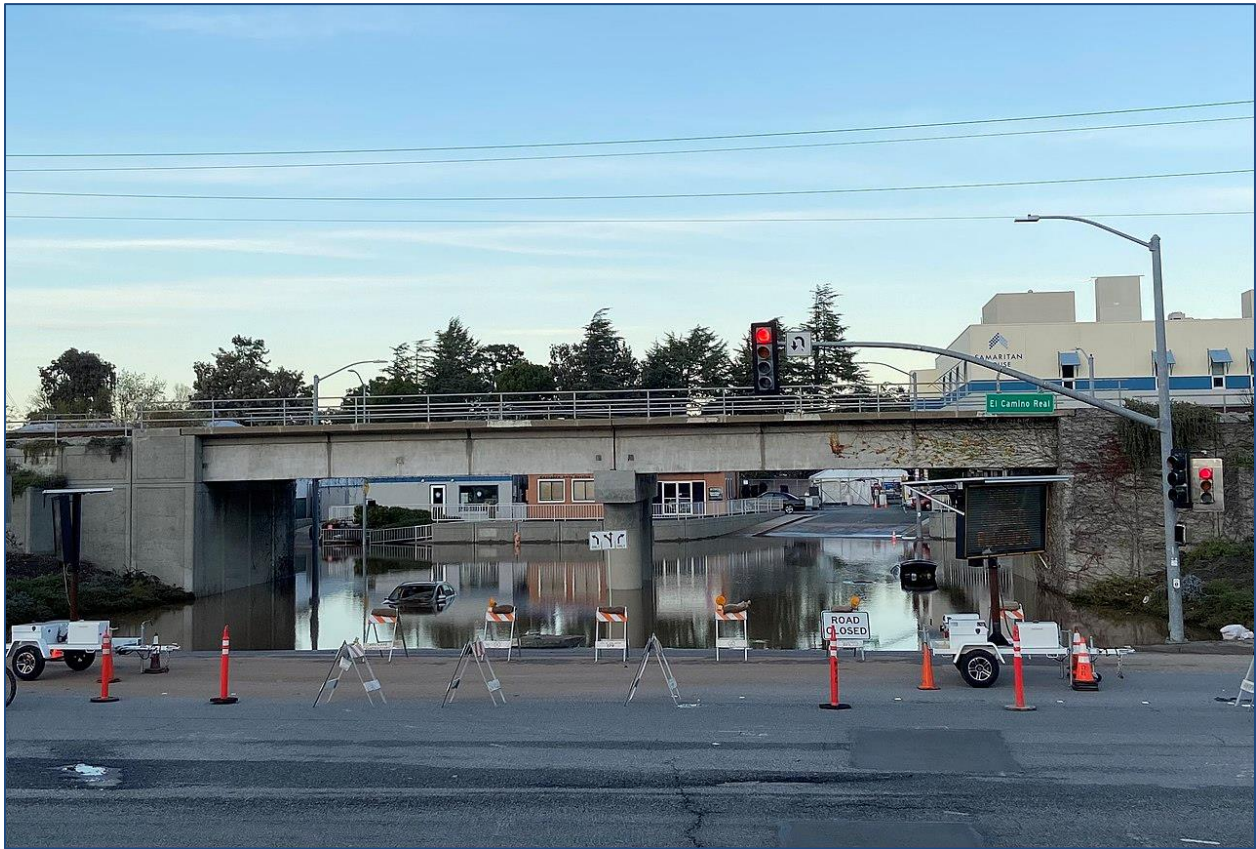
Figure B-8. Photo of pluvial flooding at an undercrossing in San Mateo, CA (Source: B. Washburn, www.flicker.com/btwashburn ; CCA 2.0)
