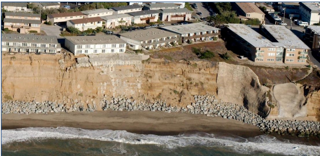
Figure 8. Photo of Esplanade Apartments threatened by cliff erosion in 2013 in Pacifica, CA. (Source: California Coastal Records Project )
