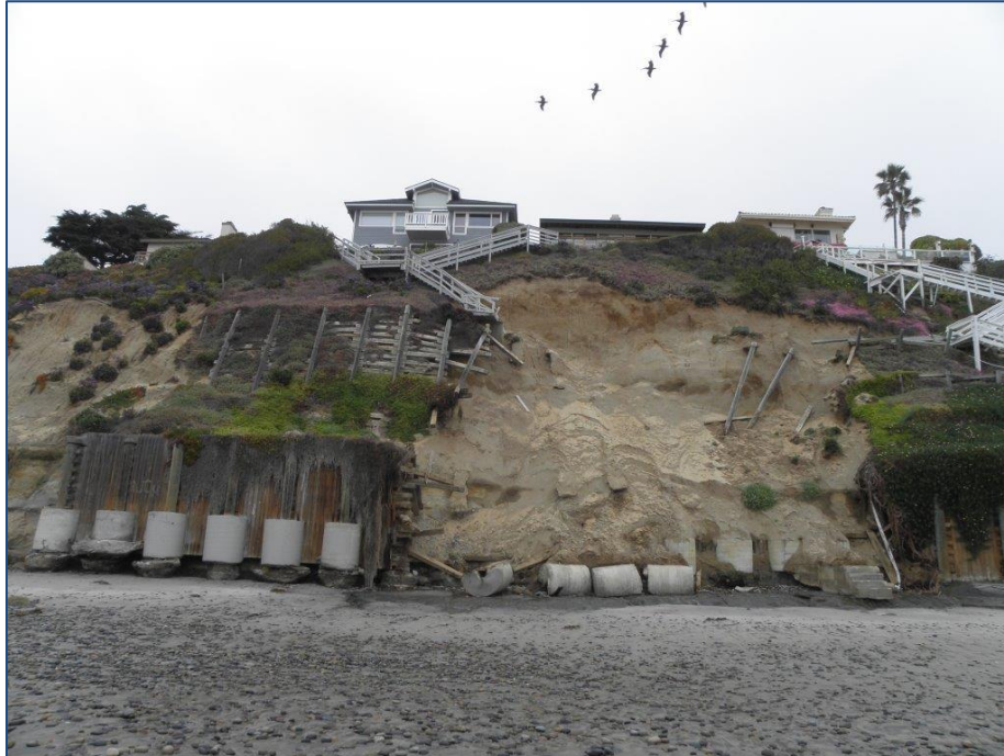
Figure 22. Photo depicting eroding bluff and exposed caissons in Encinitas, CA. (Photograph by Lesley Ewing)
