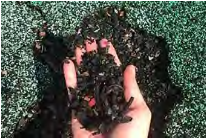
Poured-in-Place rubber playground with deteriorated top green wear layer of synthetic rubber granules exposing the base cushioning layer of shredded waste tires. (Photo: University of Massachusetts, Lowell Center for Sustainable Production)
