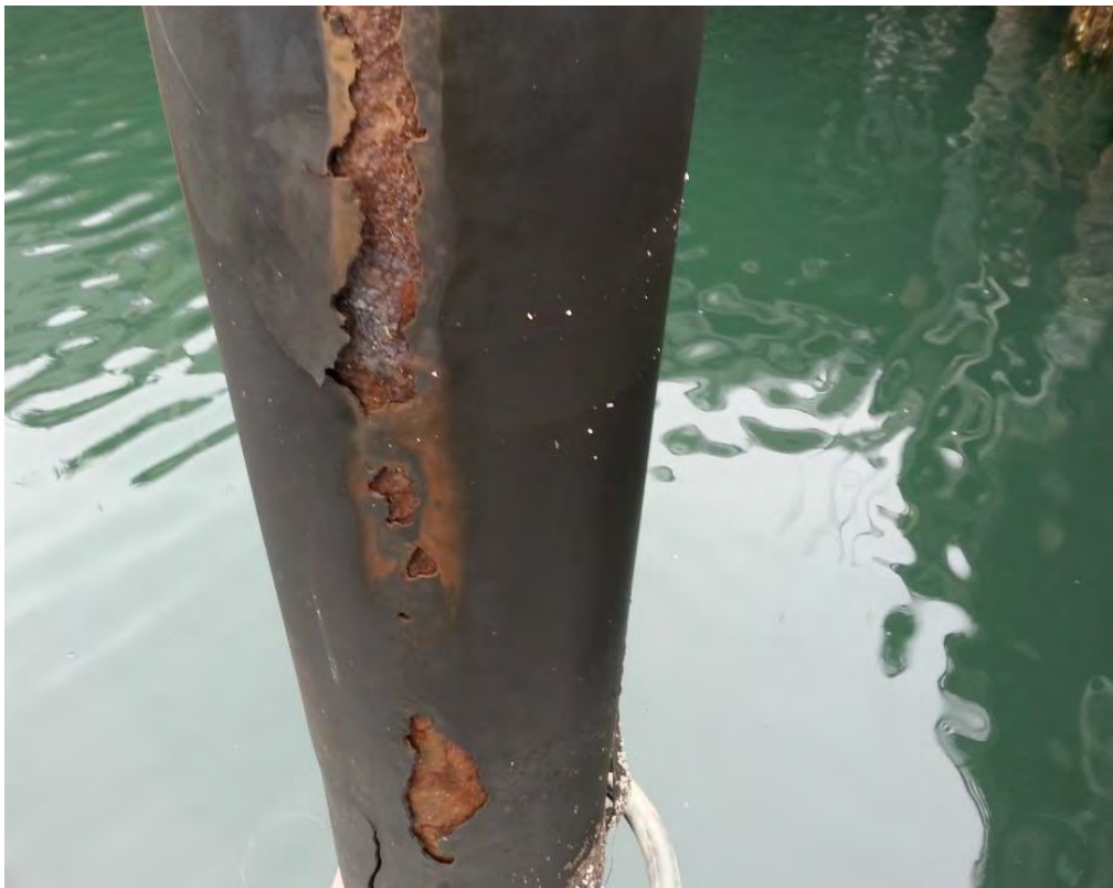
A steel dock pile with degraded vinyl pile wrap, in Santa Cruz Harbor, California. (Photo: Michael Sandeck)
