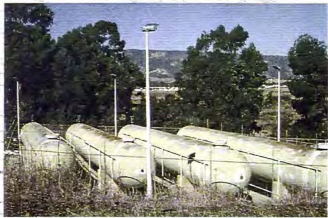
PHOTO 2 The tank farm is situated in the future location of the proposed beveledere and pedestrian trail. These tanks would be removed and the northern portion of this area would be included as part of the 5.45-acre restoration/enhancement program.
