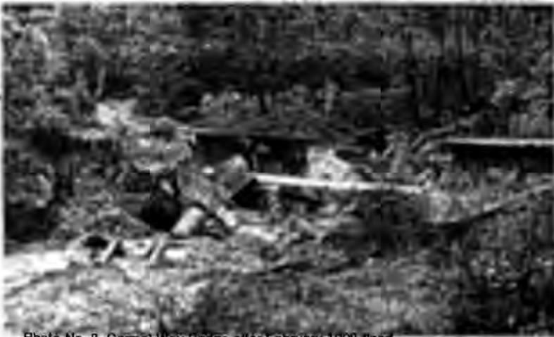
Photo No. 2 Carmel Way Bridge after February 1998 flood.
