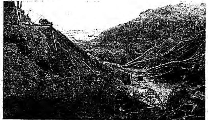
Photo No. 3 Slope failure and flood debris in lower canyon mouth of house.
