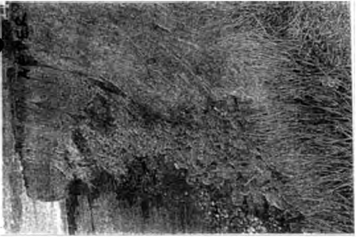
Left Photo is before Rock Placement . . . . . Right Photo is after Rock Placement
