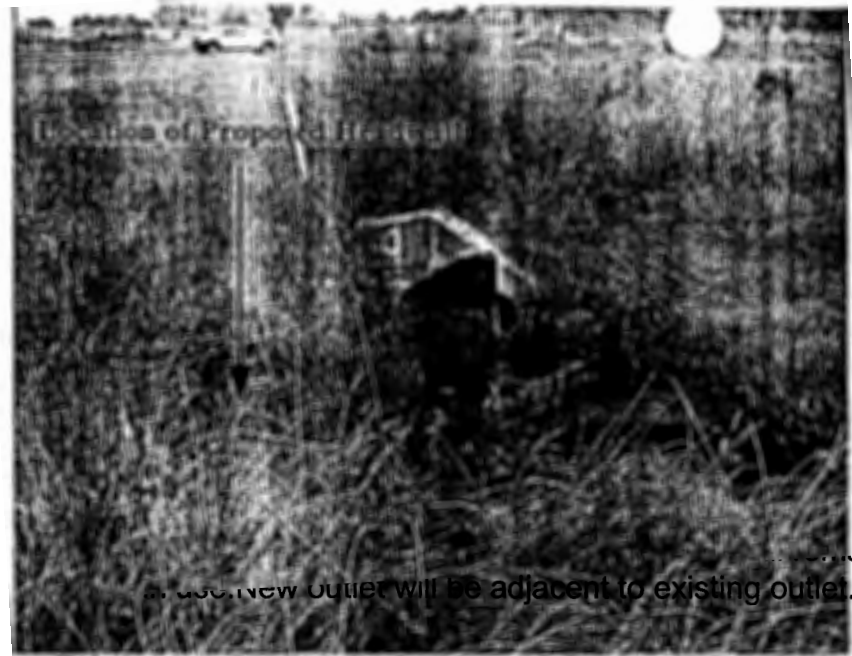
Existing headwall/outlet for Network 5 that will remain in use. New outlet will be adjacent to existing outlet.
