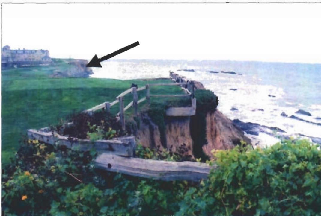
Exhibit 3b. October 2005 photo. View looking downcoast of overhanging concrete slab under tee box; remaining riprap that will be removed in summer 2006 is visible in background (arrow).
