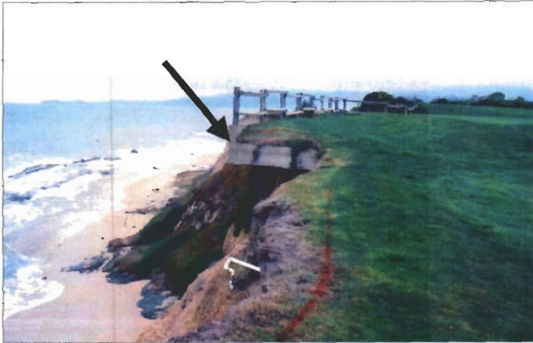
Exhibit 3a. October 2005 photo. View looking upcoast of concrete slab under tee box; slab (arrow) is overhanging the public beach below.
