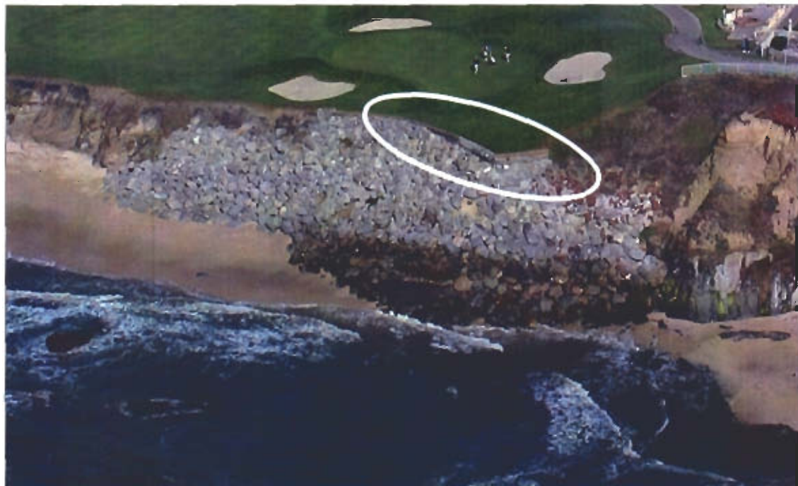
Exhibit 2b. October 2005 photo. A small portion of permitted riprap is located at the downcoast (right-hand) side of the photo; the Consent Order requires the majority of the riprap visible in this photo, and the concrete slab (edge is visible in circled white area), to be removed in summer 2006.
