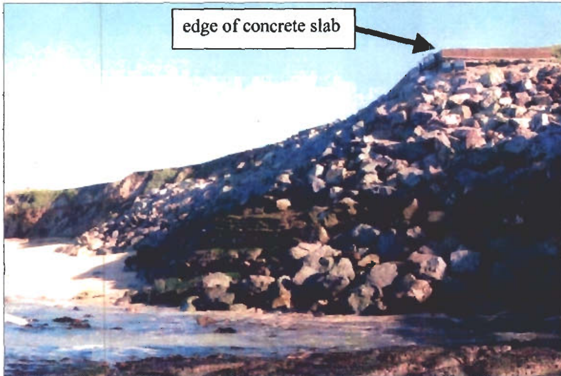
Exhibit 2a. February 2005 photo. The Consent Order that was amended in July 2005 requires Ocean Colony to remove the remaining unpermitted riprap and concrete slab in summer 2006.
