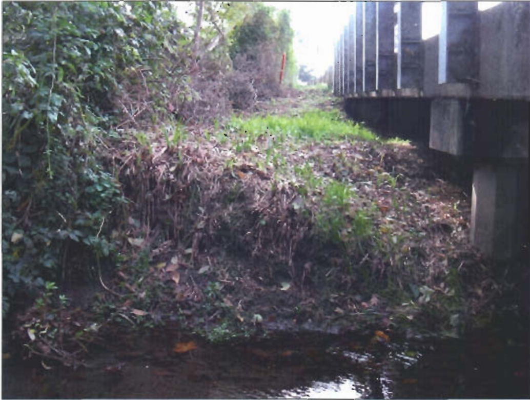
View of sediment accumulation on the left bank on the upstream (southern) side of the bridge.
