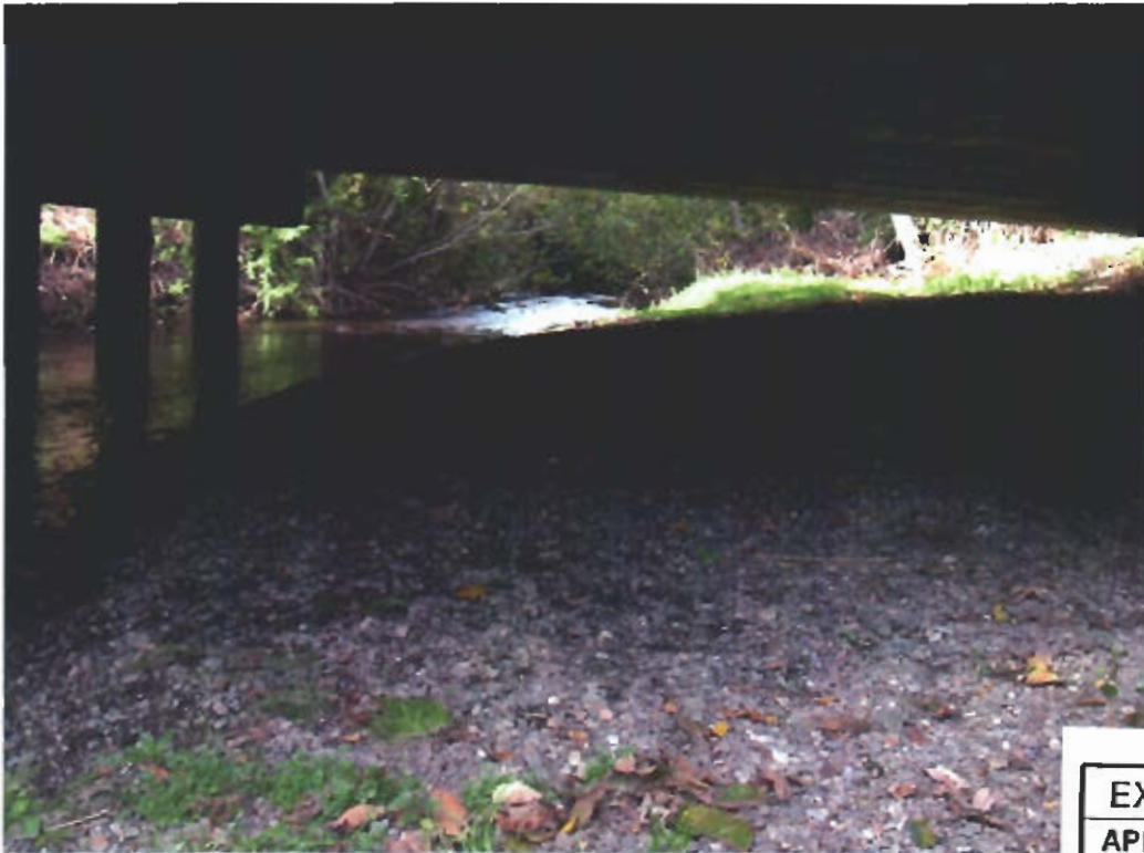
View of sediment accumulation beneath the bridge, looking downstream.
