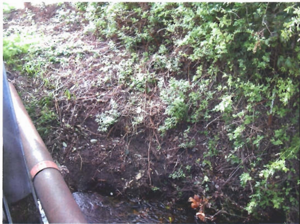
View of sediment accumulation on the left bank on the downstream (northern) side of the bridge.
