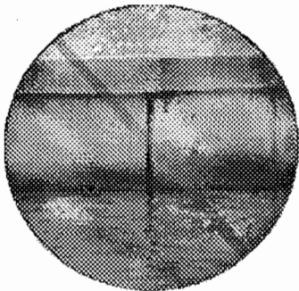
Concrete panel corners are difficult to lock. This brand new concrete panel wall has already lost its integrity.
