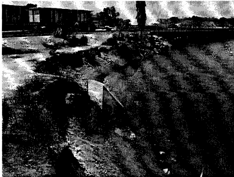
Figure 2: NCTD Bridge 243.0 Southeast Abutment Looking Downstream to the west towards the bridge; this is the project area to be excavated
