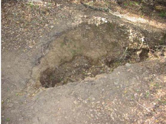
Erosion occurring along existing road
