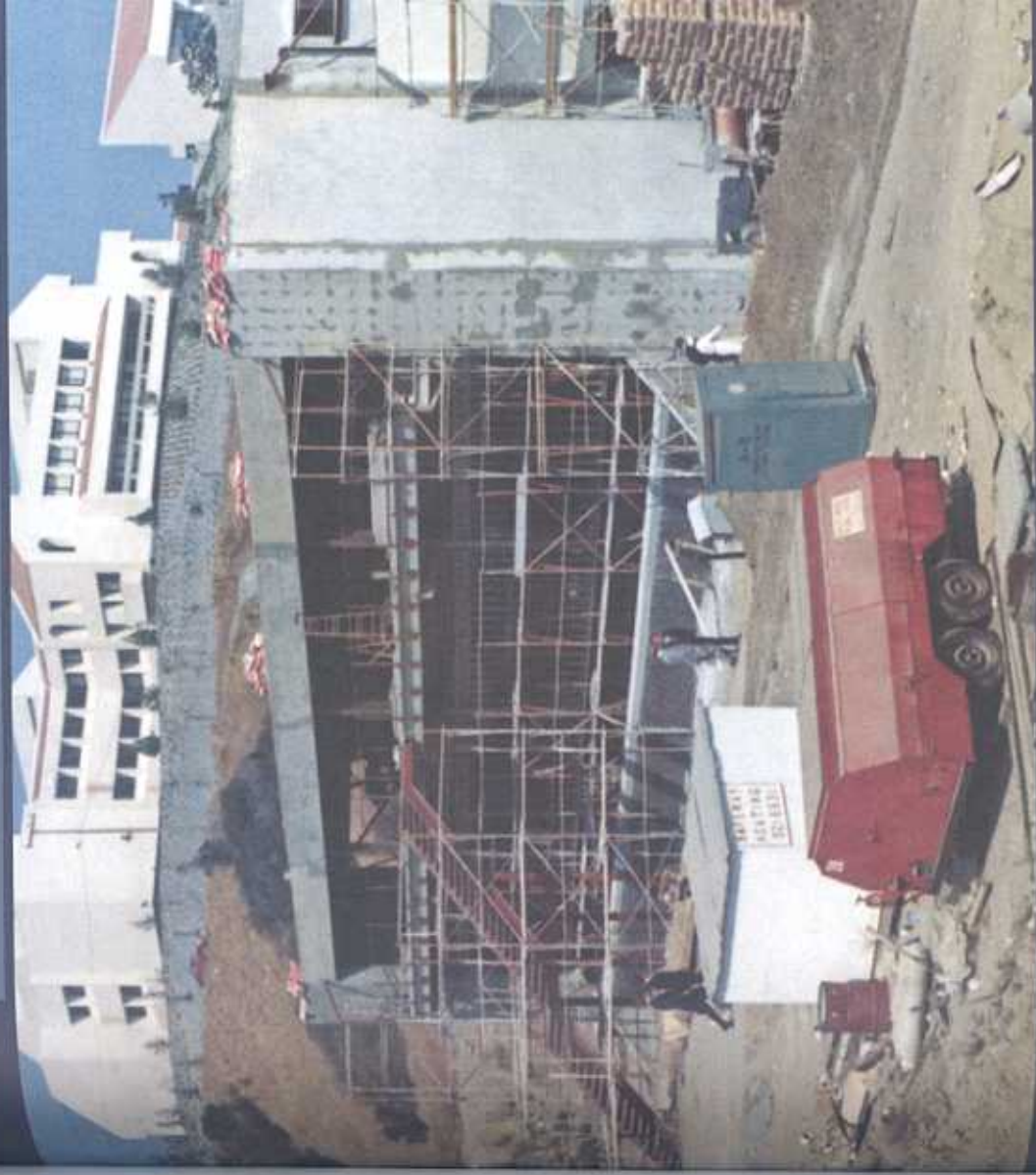
In 1972, with school in Malibu already open, Firestone Fieldhouse sprints toward its 1973 completion. In the foreground dust, the Raleigh-Runnels Memorial Pool has not yet begun.
