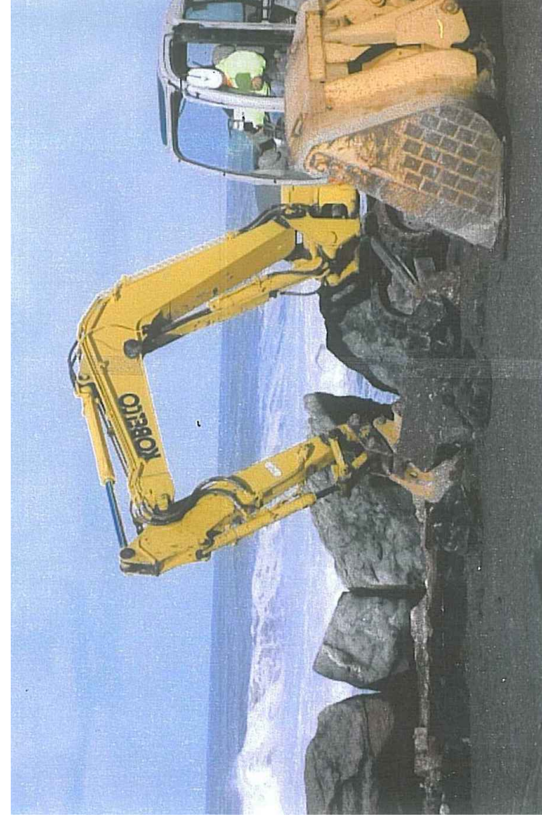
Loader and Backhoe Used to dig out slump hole and replace rock. All work was done from the parking lot
