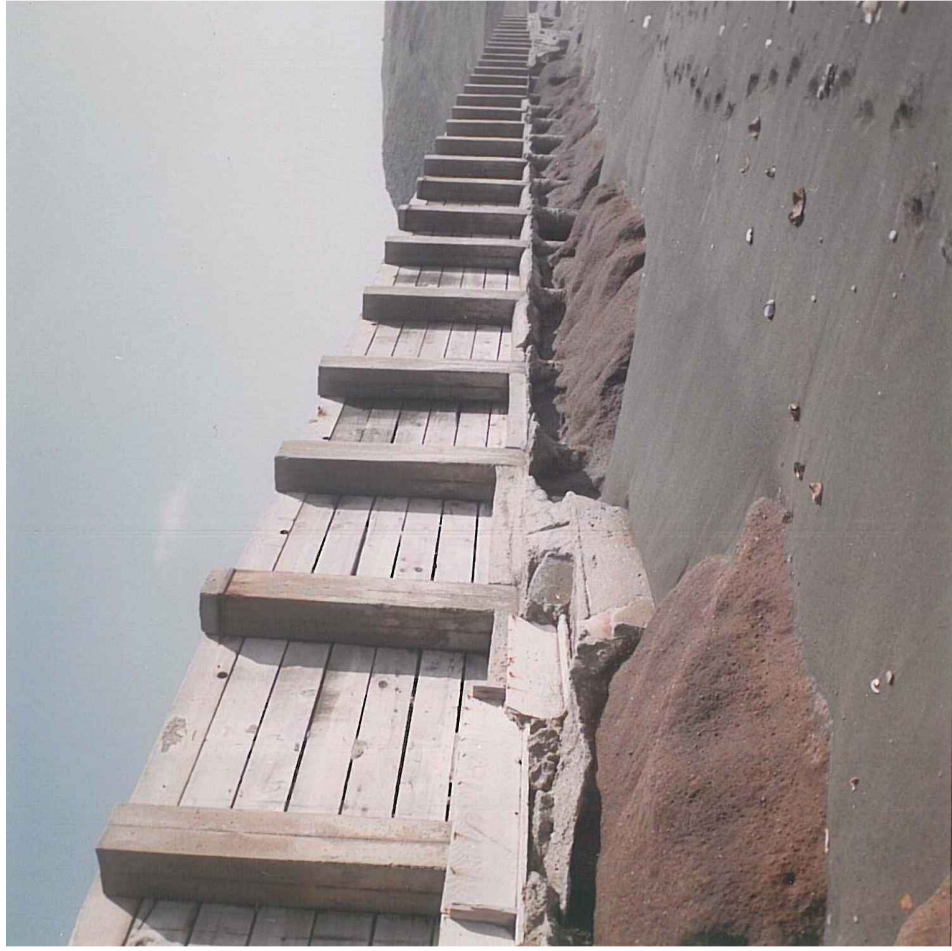
ORIGINAL WALL BEGINNING TO ERODE IN 1965
