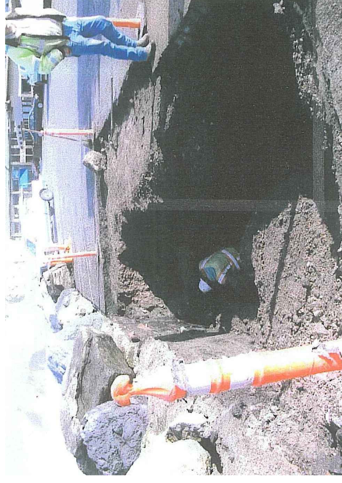
Part of Sink hole being dug out worker cleaning out Hole. (10-15 Feet deep)
