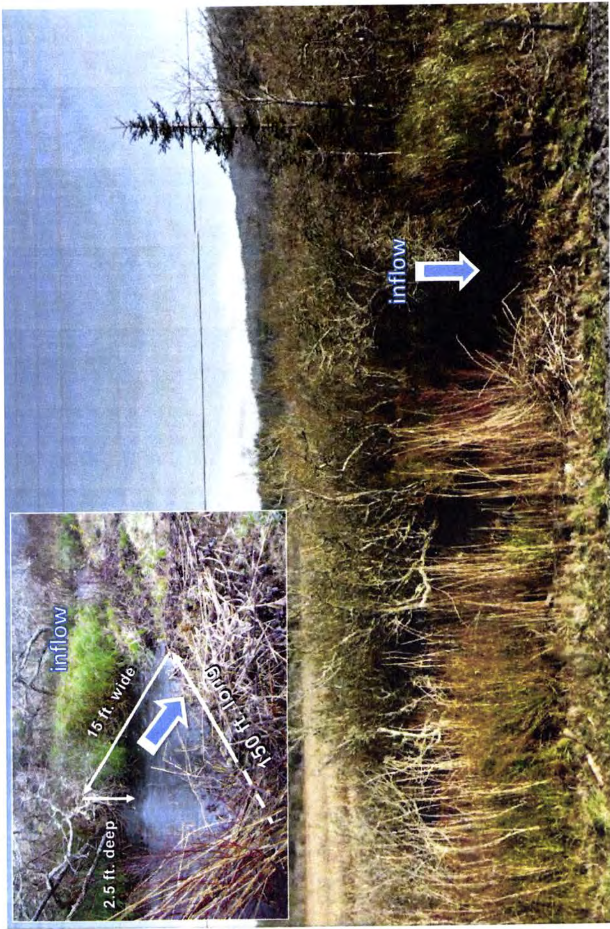
Figure 6. Encroached and partially plugged entrance to Southern Culvert (#MP24.46); inflow passes under Highway 101 to beach. No trees will be removed. Excavator will remove muck soil and associated live and decomposed vegetation currently choking entrance to culvert. All excavated material will be removed and hauled to an approved disposal site by Caltrans. A very small amount of cattail, rush, and live/decadent willow scrub (<3 inches dbh) will be removed along ditch and at entrance to culvert.
