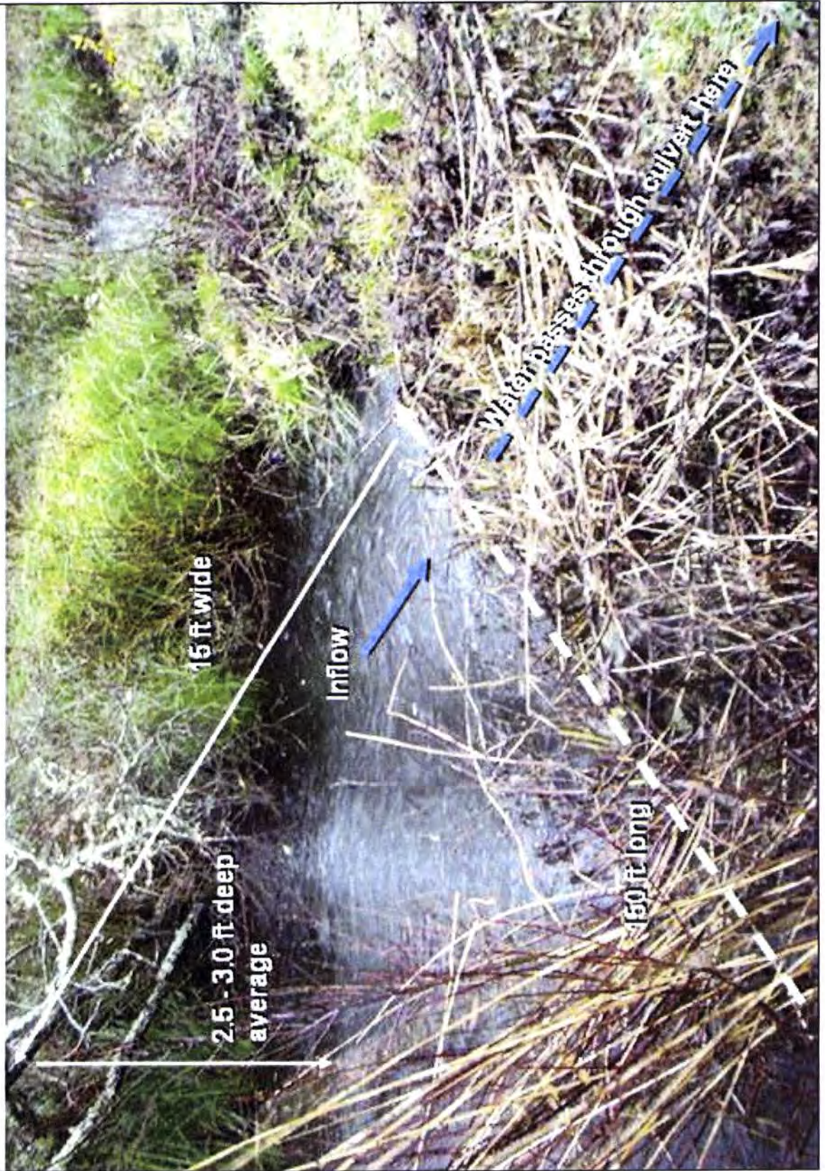
Figure 7. Inflow at ditch draining into Southern Culvert (#MP24.46); water passes into culvert and under Highway 101 to beach. Extent of excavation is indicated. There are no special status plants within the ditch excavation area. No trees will be removed. A small number Wolf's evening primrose ( Oenothera wolffii ) CNPS list 1B, in road shoulder will be impacted by excavator (David Imper pers. comm. Service 2011).
