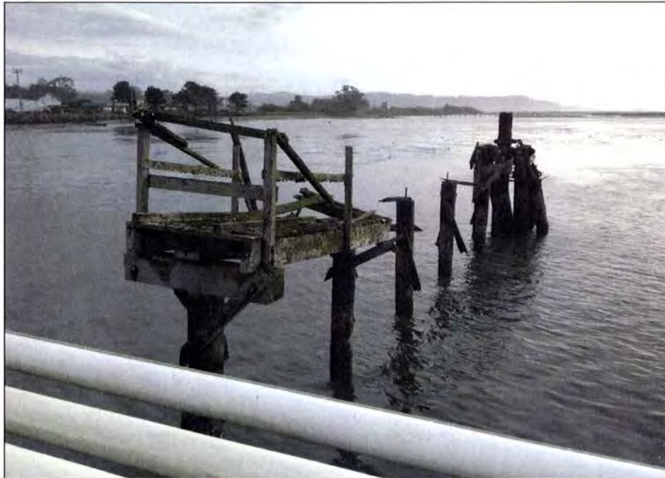
Photo 12. Structures South of the Trestle That Will Be Removed in 2015 as Mitigation (View Looking South from the Trestle)
