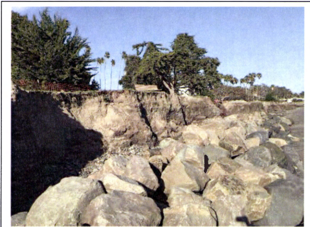
Overtopping of the existing permitted rock revetment eroded landward park area and required importation of cobble to stabilize the eroded gap between the rock revetment and the eroded park area.
