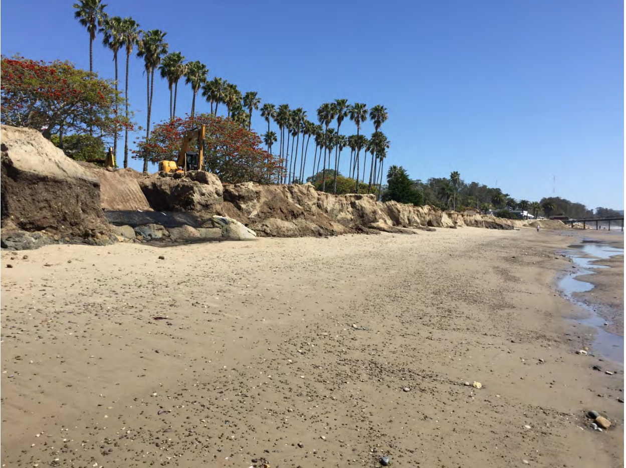
The above photograph shows the central area of Goleta Beach County Park after erosion occurred in March of 2016.
