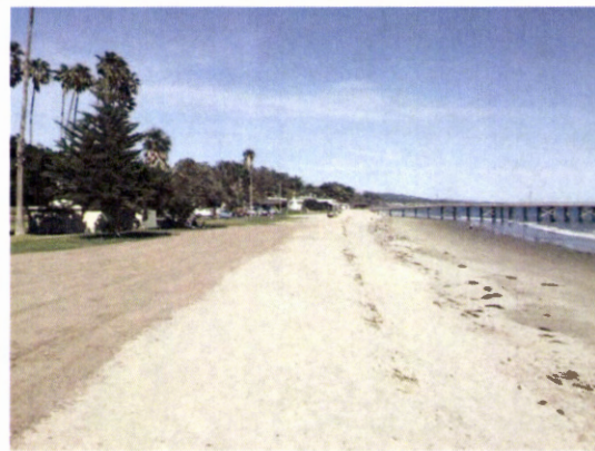
Areas subject to emergency repairs have now been covered with sand by both natural spring time accretion and heavy equipment.
