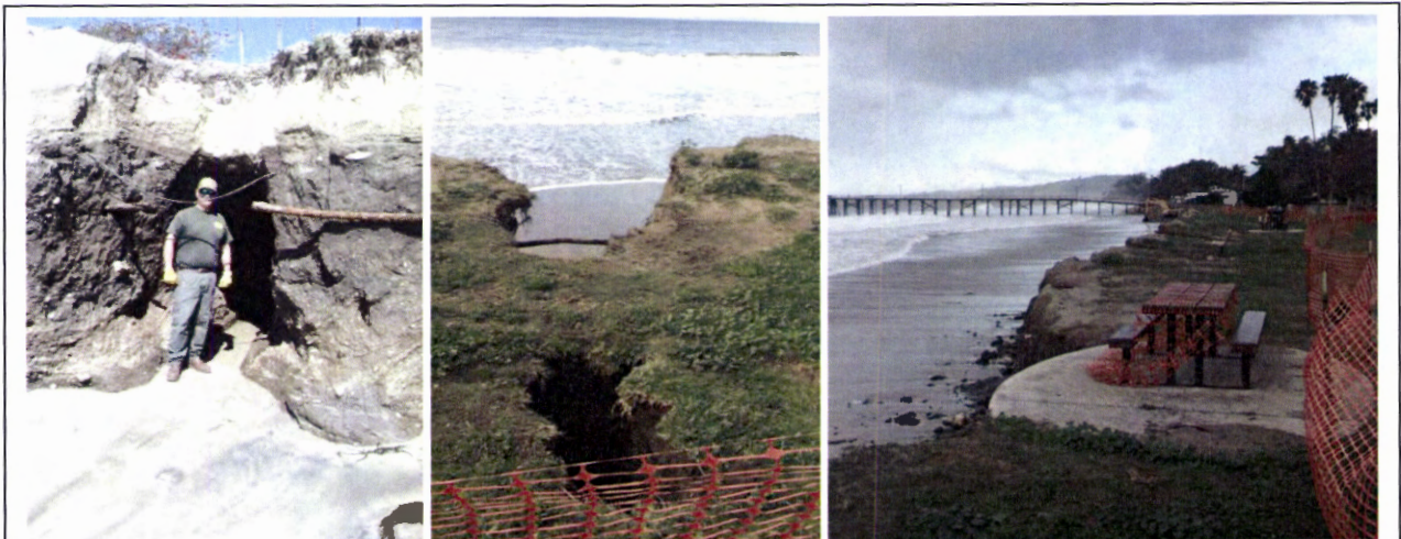
Sink holes that developed in March 2016 exceeded more than 10 feet in depth in some locations (left), with crevasses extended 15-20 feet deep into the lawn resulting in imminent substantial impacts to public safety at the park. The County took permitted emergency action to cordon off and fill these areas and to initiate repairs.
