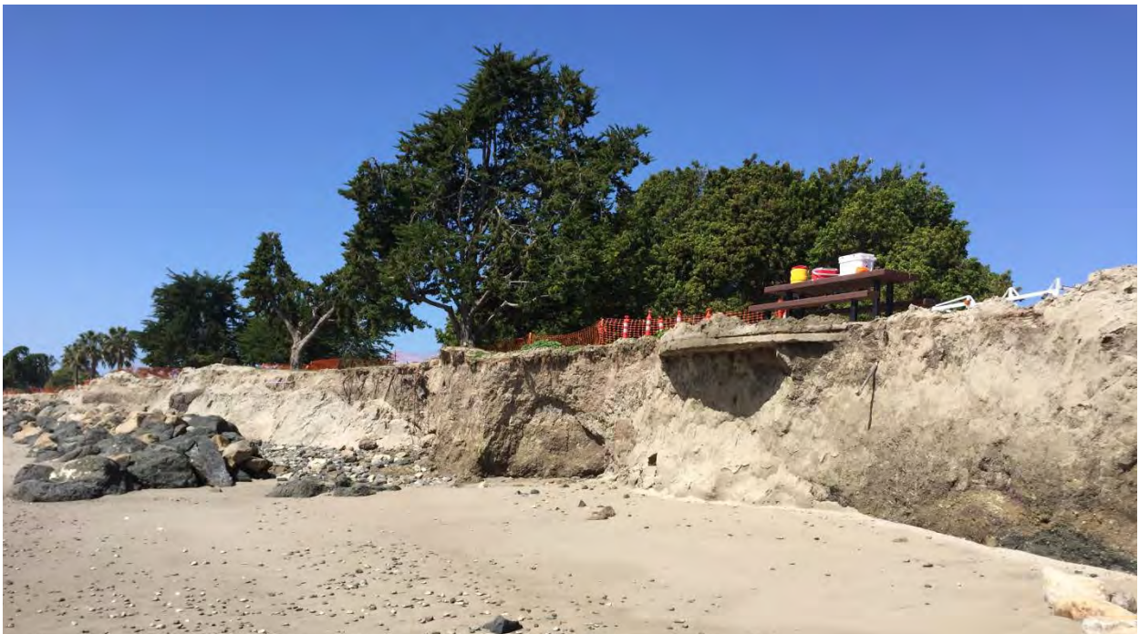
The above photograph shows a portion of Goleta Beach County Park after erosion occurred in March of 2016. On the left side of the photograph is the exposed rock revetment and on the right side of the photograph is a picnic table area that was undercut by wave caused erosion.
