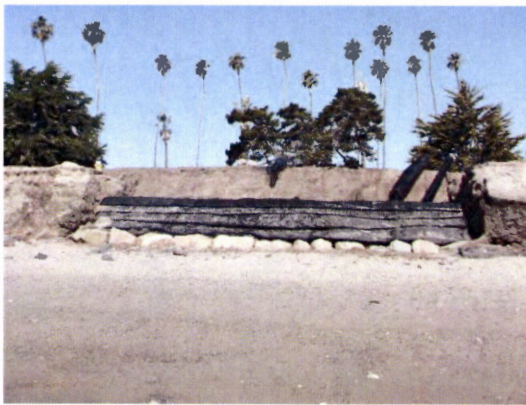
In response to damaging erosion, work crews installed geotextile fabric earth filled cells to protect park facilities in areas that were not already protected by the existing revetment (boulders were temporary and have been removed).
