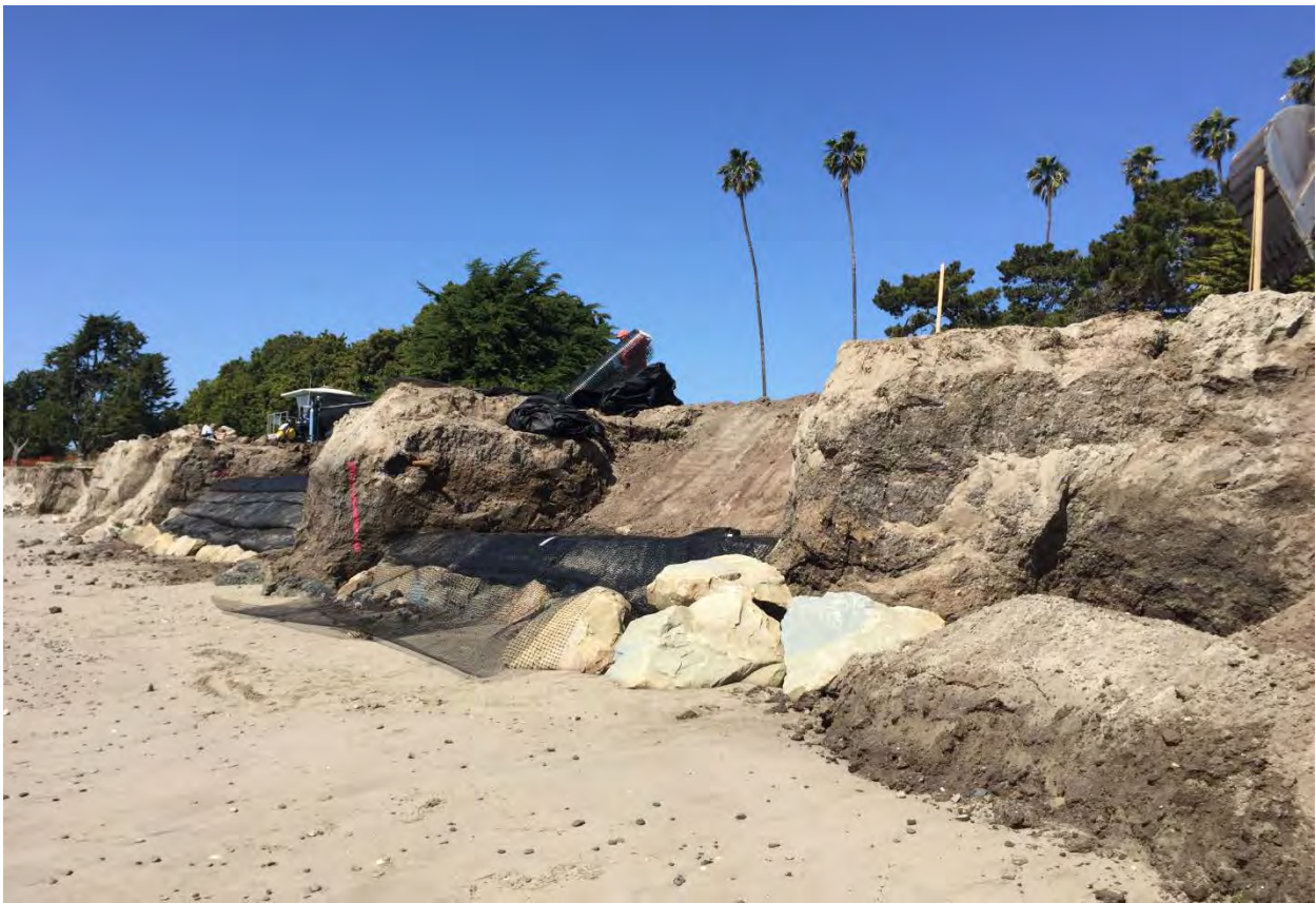
The above photograph shows installation of two segments of the geotextile cells.
