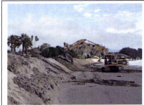
Following completion of the sand berm in December, frequent maintenance involved use of excavators to rebuild the eroding sand berm.
