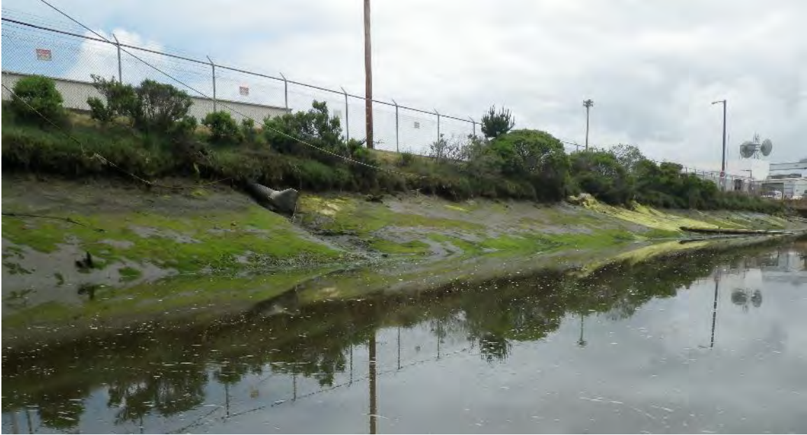
Figure 6. Culvert connecting the Frog Pond Stormwater Detention Basin and the Intake Canal.
