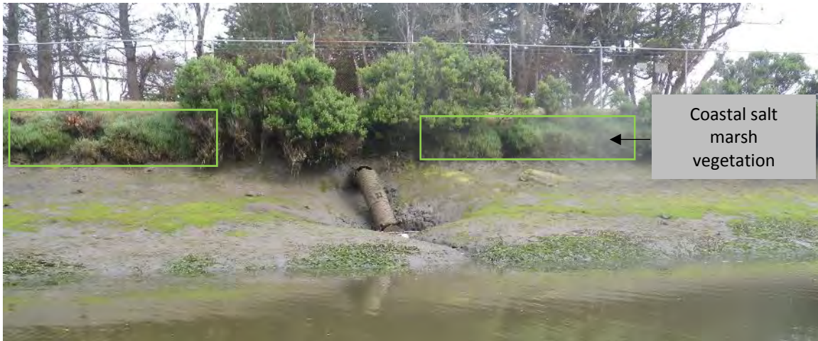
Figure 3. Downstream end of the culvert connecting the Buhne Point Wetlands Preserve and the Intake Canal. Coastal salt marsh vegetation is indicated in green boxes.
