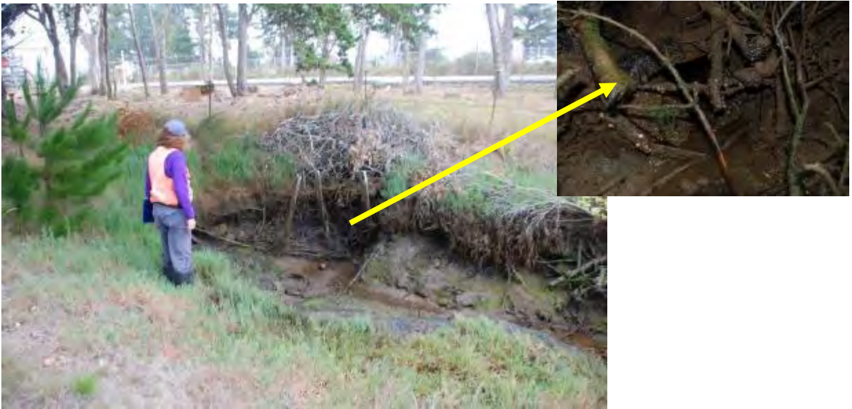
Figure 7. Upstream end of the culvert connecting the Buhne Point Wetlands Preserve and the Intake Canal.
