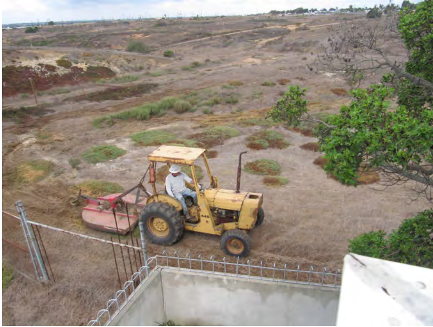
Mowing and scraping near the eastern site boundary on October 11, 2012. This mowing was taking place within 100 feet of existing residences, as permitted and required, but similar actions that were not permitted took place across a much larger area (see map on previous page). Source: Banning Ranch Conservancy.
