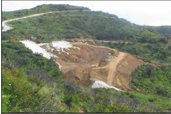
Area of unpermitted grading that will be restored pursuant to a Commission enforcement action.
