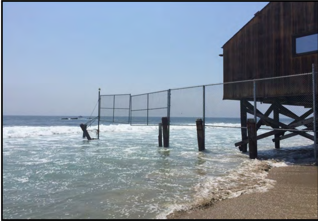
Exhibit 3: Section 30821 was utilized to remove many impediments to public access and recreation, such as this private fence in Malibu Lagoon State Beach.
