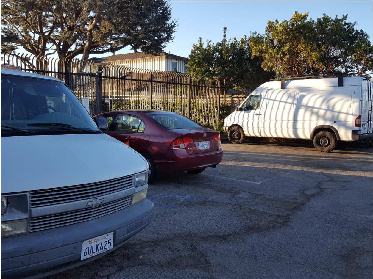
Fence/ Parking Area in 2018 (Note: No ADA Parking Signage and ADA striping is faded):
