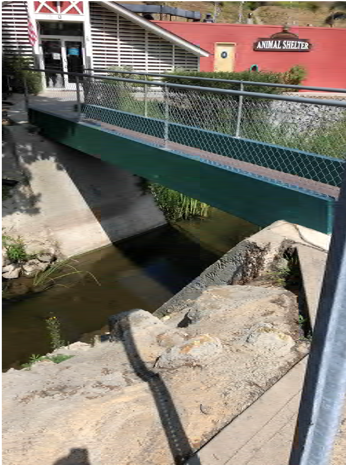
Figure 4. The pedestrian bridge crossing Laguna Canyon Creek between the parking lot and the City of Laguna Beach Animal Shelter.
