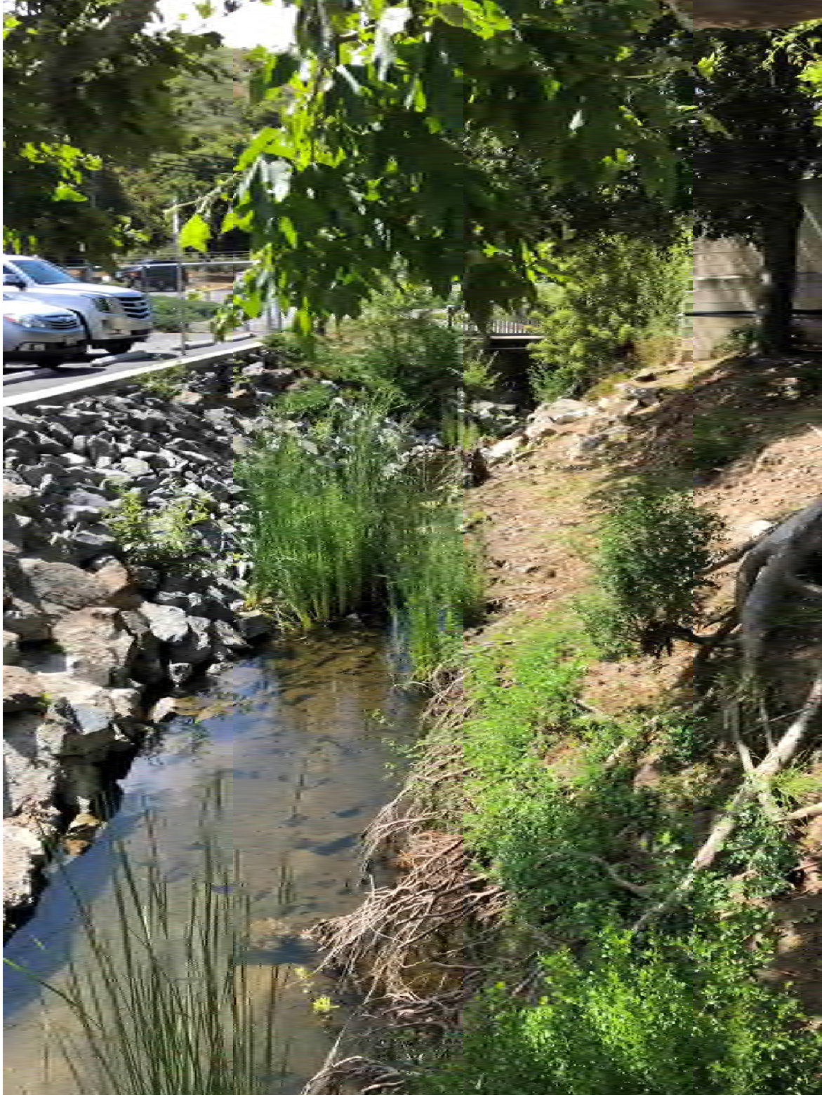
Figure 2. The banks of Laguna Canyon Creek adjacent to the City of Laguna Beach Animal Shelter lined with loose rip rap, concrete lined rip rap, and bare dirt.
