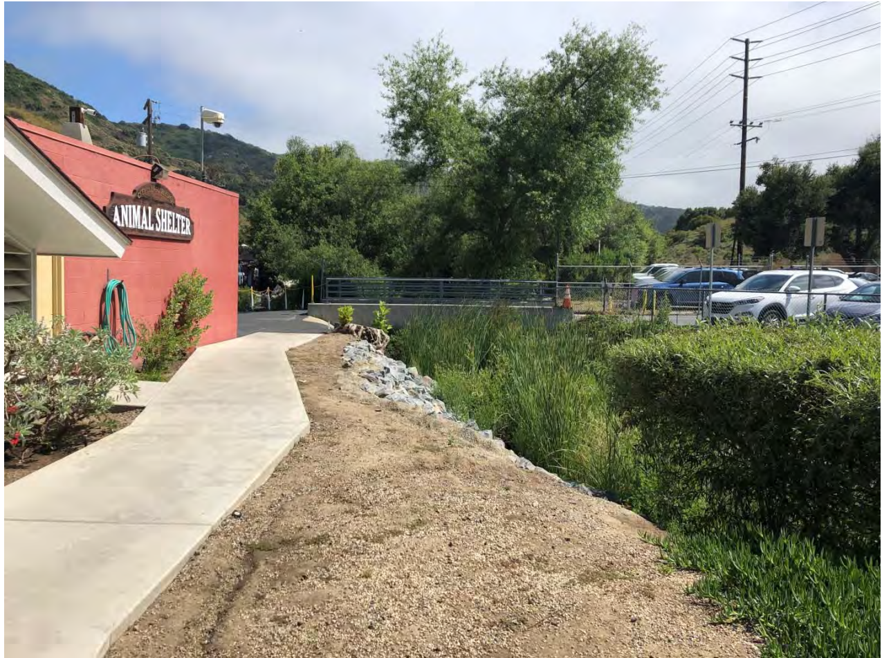
Figure 1. The eastern bank of Laguna Canyon Creek adjacent to the City of Laguna Beach Animal Shelter lined with loose rip rap and bare dirt.
