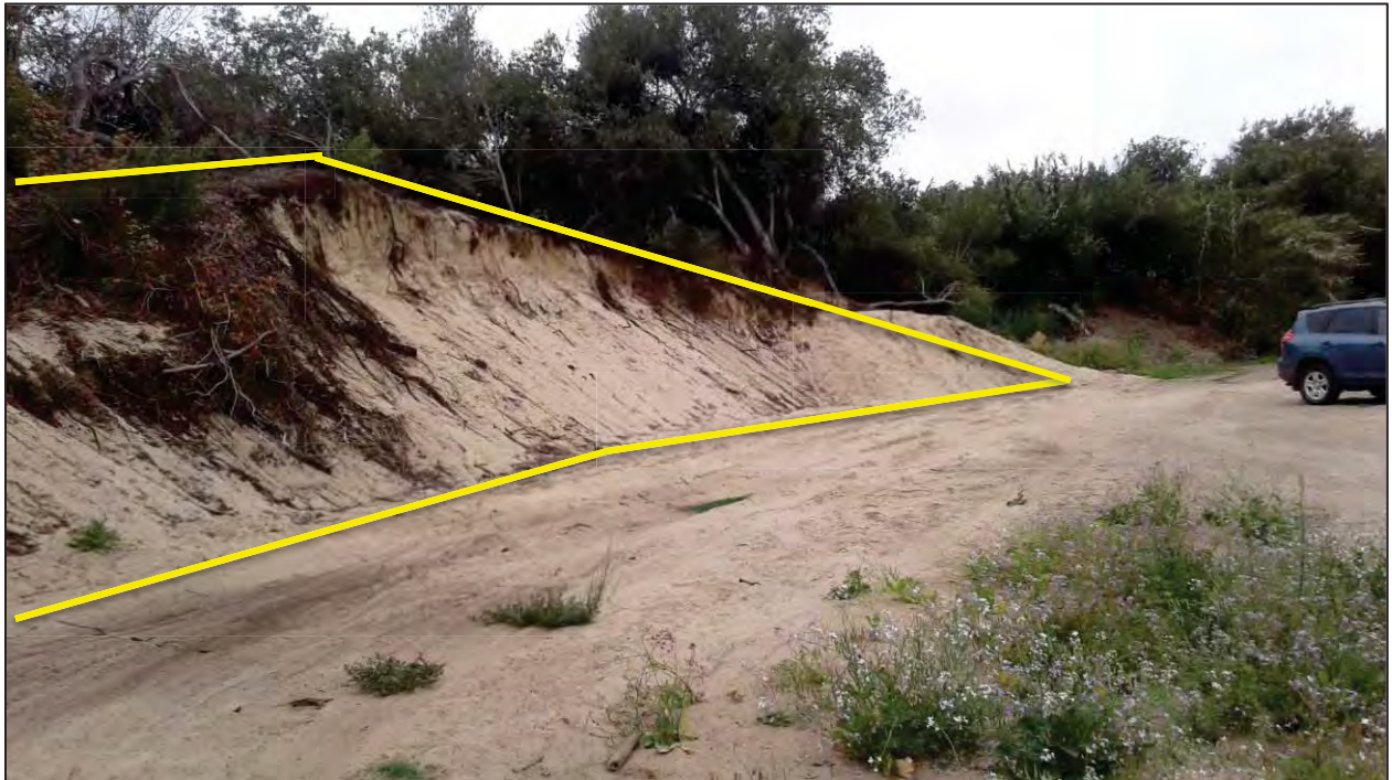
Photo 1. View of the slope that was graded along the west boundary of the site and where restoration is proposed (i.e., native seeding and planting, jute netting and straw wattles).
