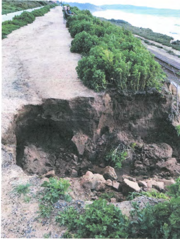
Figure 4: Upper Bluff Slope Failure Below 7 th Street
