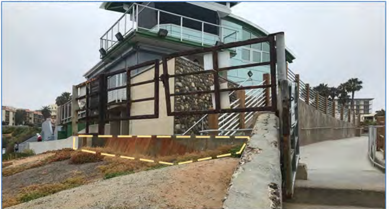
Gate with retaining wall (outlined) constructed underneath, looking south towards Coast Blvd.
