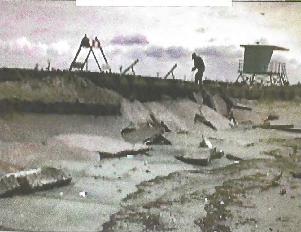
CLAREMONT LAUNCH RAMP EROSION
