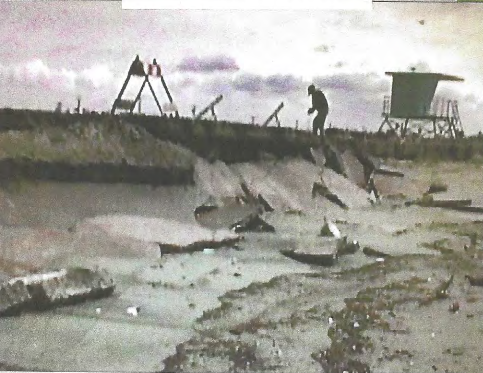
CLAREMONT LAUNCH RAMP EROSION
