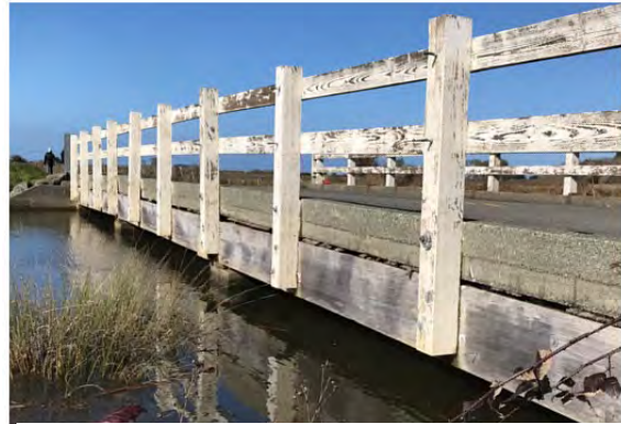
Figure 8. Upstream of existing bridge when levees overtopped and adjacent fields flooded (photograph taken by Commission staff during king tide on February 8, 2020).
