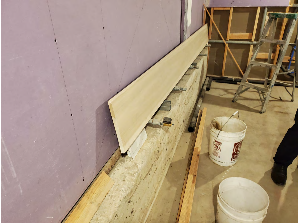
New gas line and valves in proposed kitchen area (Photo taken 4/16/21)
