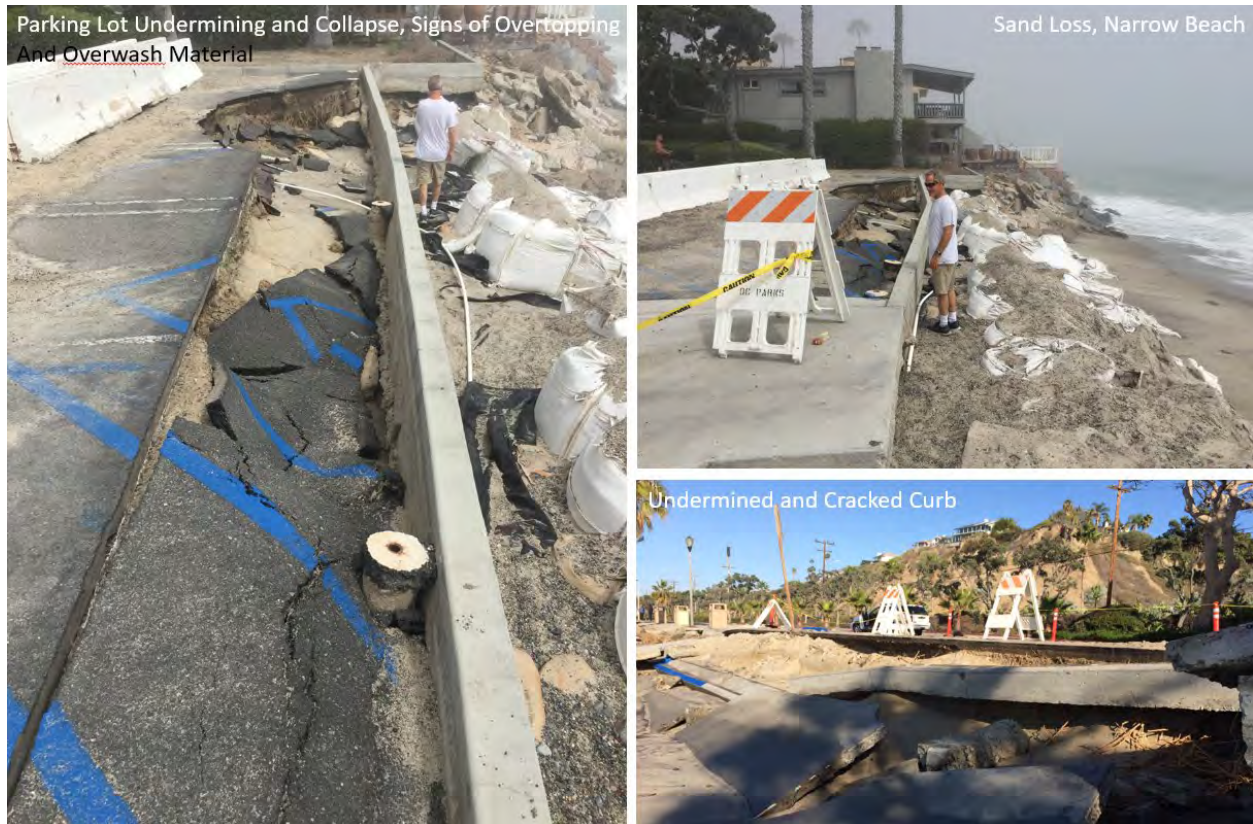
FIGURE 2-1. SOUTH REACH – DAMAGED PARKING LOT AND ERODED BEACH CONDITIONS
