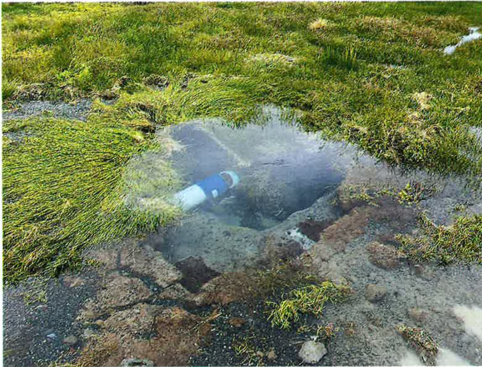
4/19/22 – Emergency Repair Location – See broken/detached pipe in self-excavated hole
