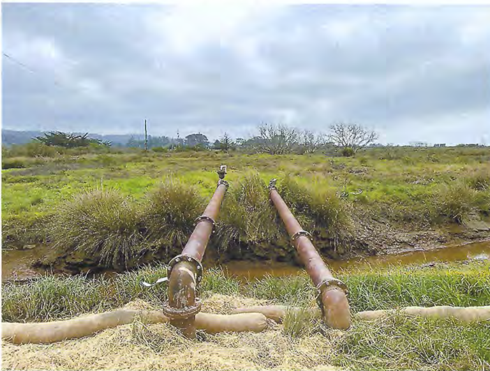
4/25/22 – Emergency repair site #2 is located on far side (west side) of left (southern) pipe and emergency repair site #3 is located on the near side (east side) of right (northern) pipe.
