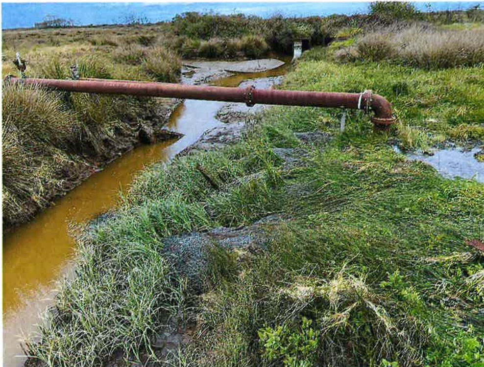
4/19/22 – Emergency Repair Location – See displaced gravel
