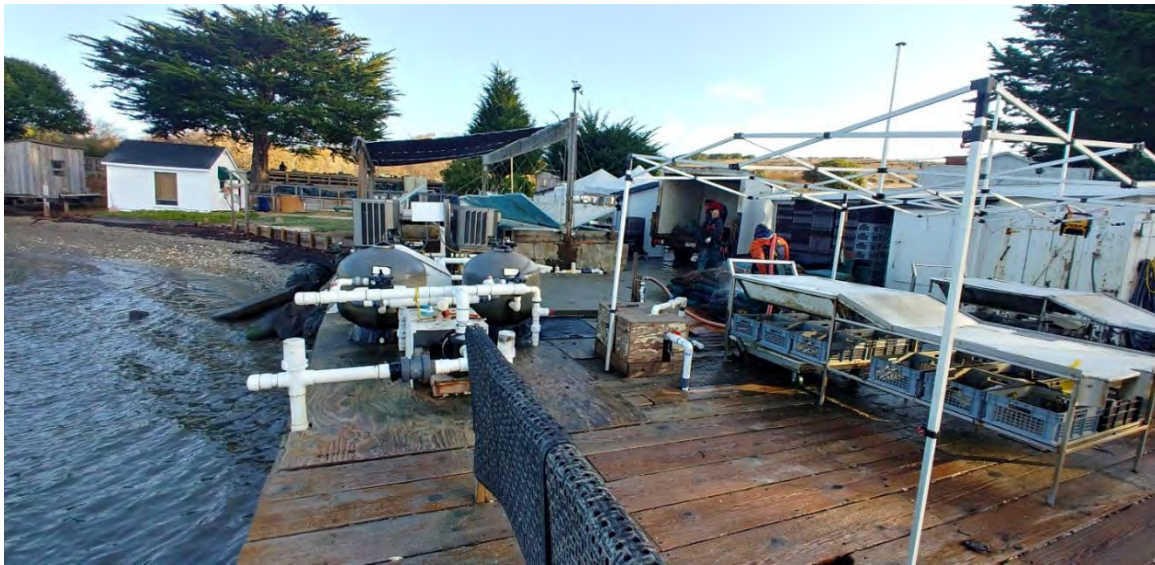
Figure 3: View on landward end of pier looking towards the wet holding system, the plumbing rising through the dock on the left is the main water intake line for the system.
