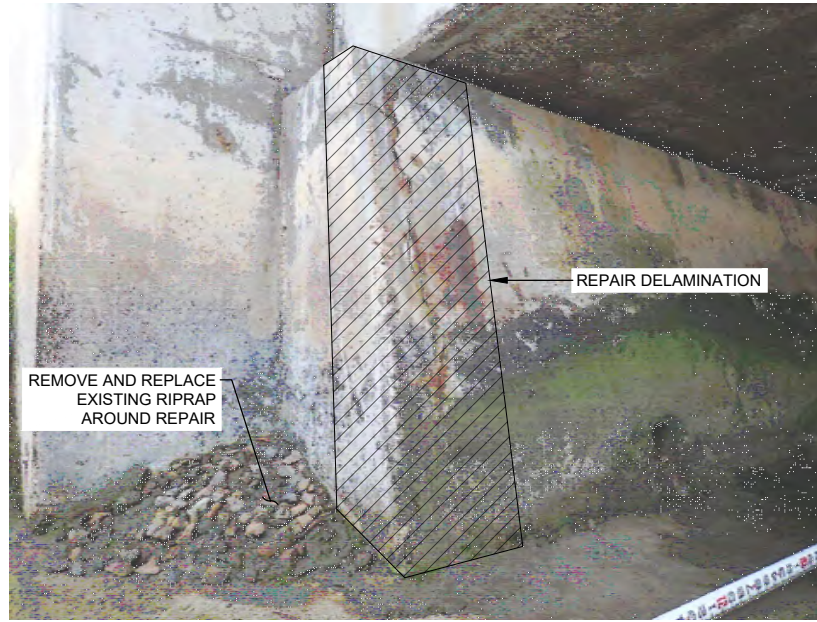
PHOTO 2 CLOSED CORROSION SPALLING AT SOUTHWEST CORNER AT ABUTMENT 1, LOOKING NORTH
