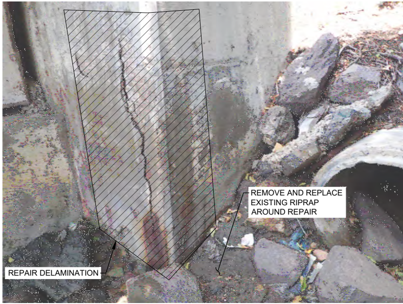
PHOTO 1 DELAMINATION AT NORTHWEST WINGWALL AT ABUTMENT 1, LOOKING WEST
