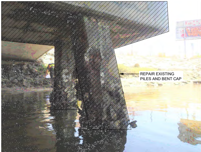
PHOTO 4 OPEN CORROSION SPALLING AT THE TOP OF PILE A9, LOOKING SOUTHEAST
