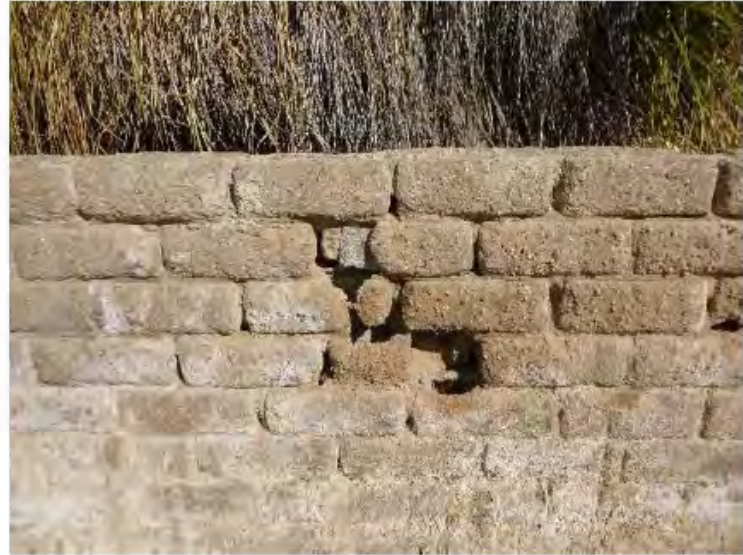
Degradation of existing wall
