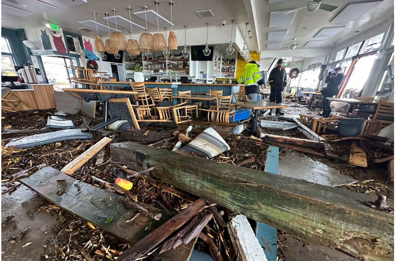
Figure 6 Piece of Capitola Wharf deposited inside Zeldas restaurant (Credit: Shmuel Thaler)
