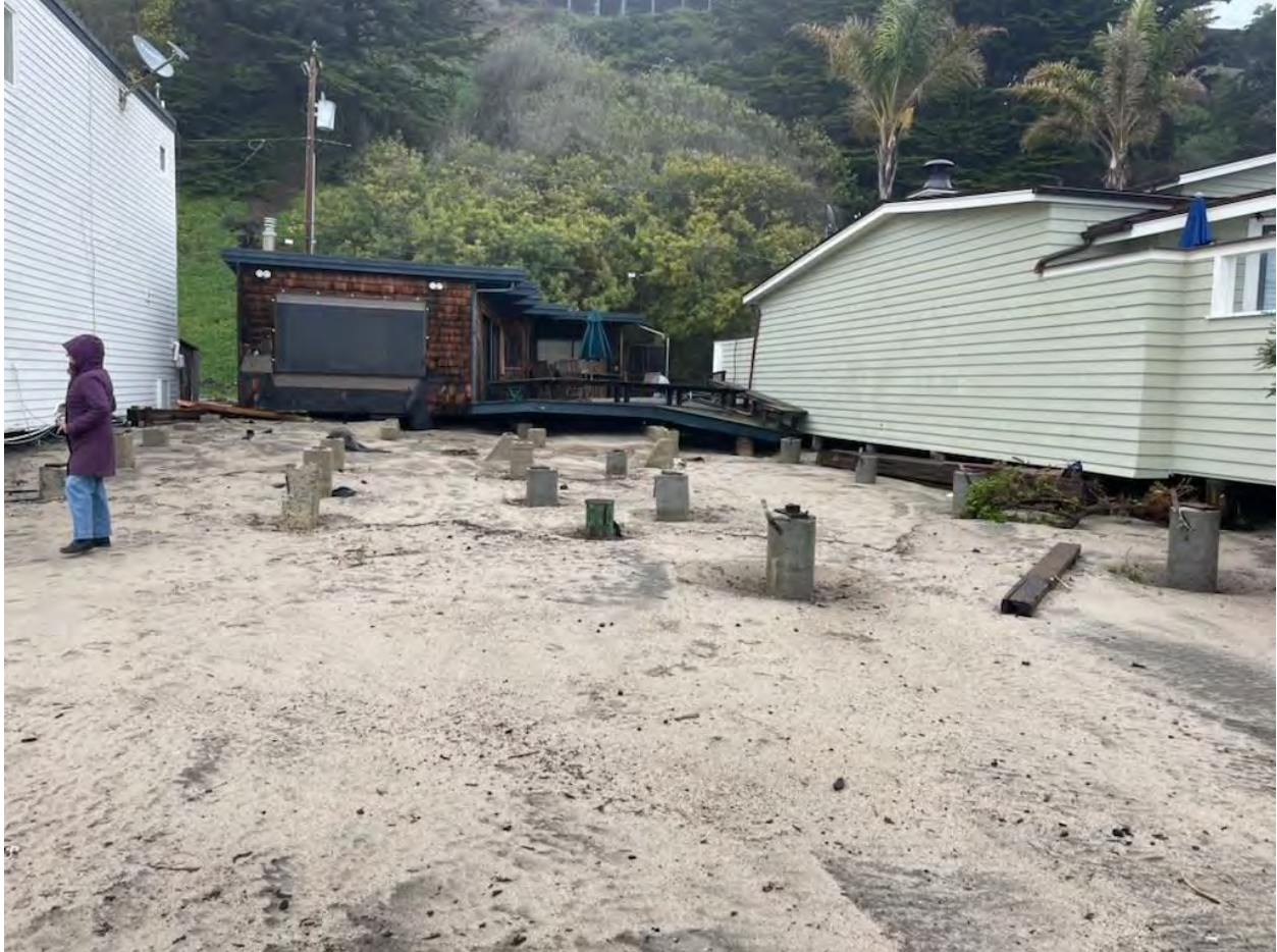
Figure 1 Beach Drive house displaced off its foundation (Credit: Santa Cruz County Sheriff's Office)
