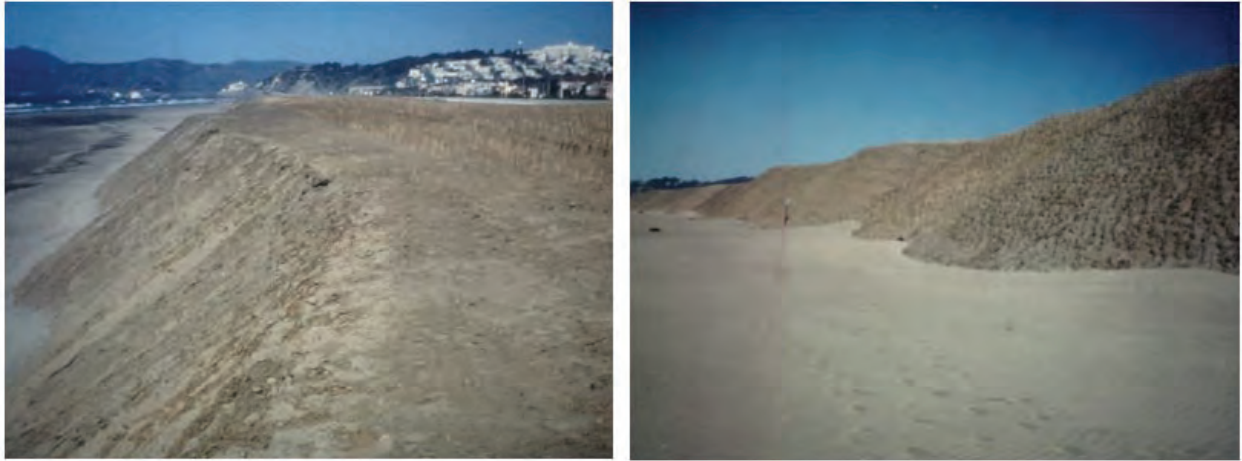
Figure 2-3: The newly constructed and planted Ocean Beach artificial foredune ridge in March 1985, with incipient dune sand accretion confined to the toe of the steep seaward slope.
