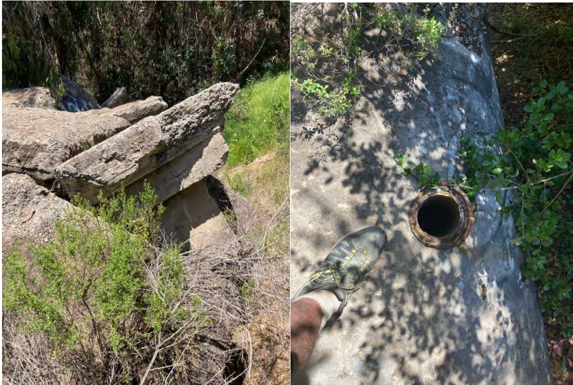
Figures 2 and 3- concrete footings (25+) and fill port for the underground storage tank. These conditions are hazardous to children playing nearby.
