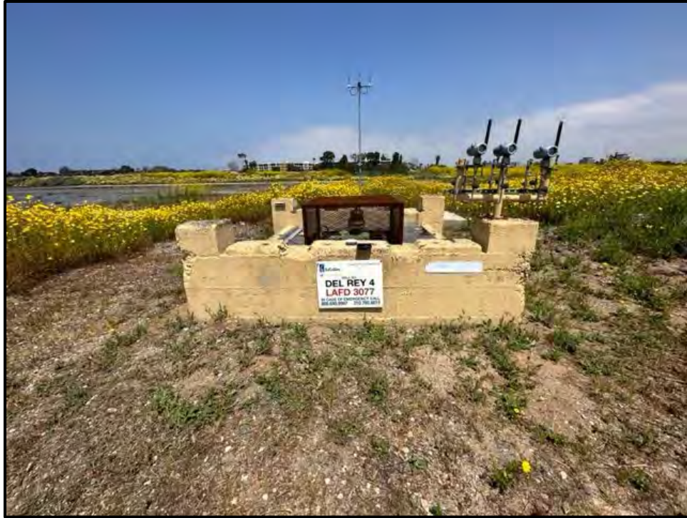
Figure 5: View of the DR-4 well facilities, facing northwest.
