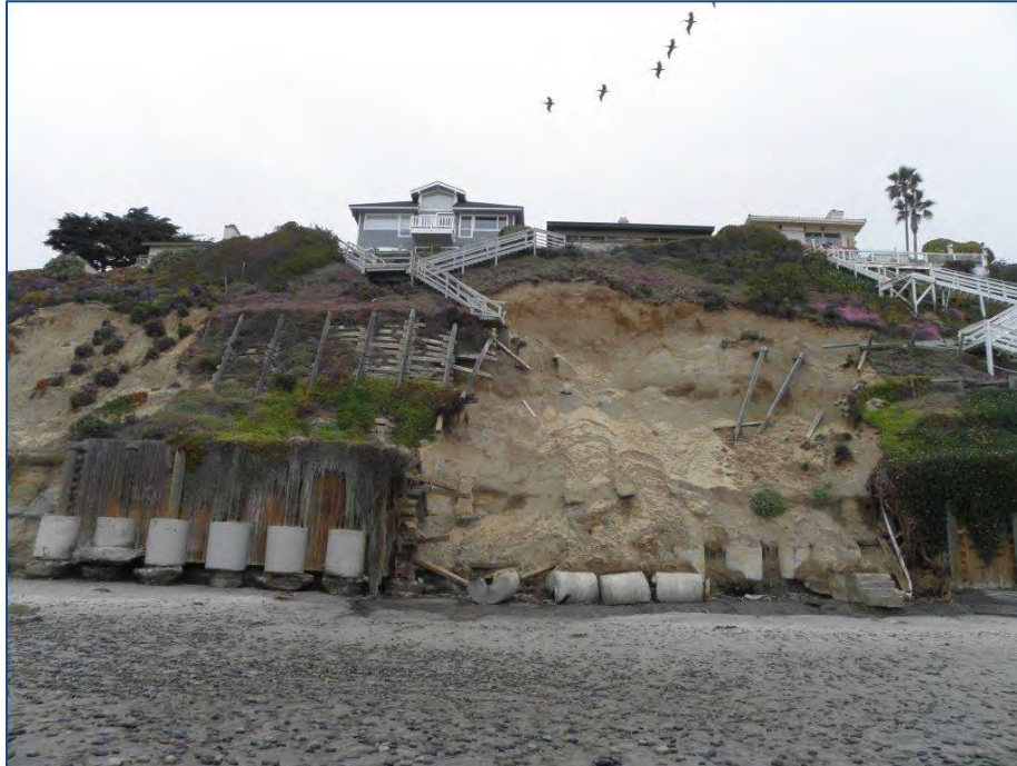
Figure 22. Photo depicting eroding bluff and exposed caissons in Encinitas, CA. (Photograph by Lesley Ewing)
