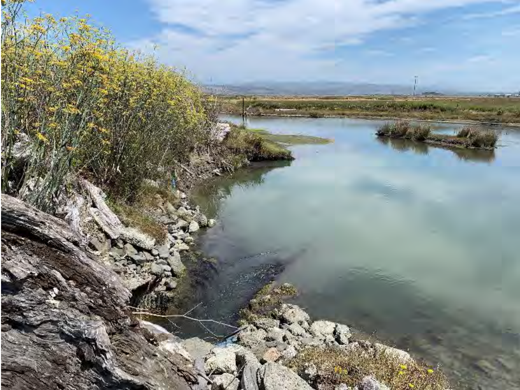
Photo 13—Failed culvert on inboard side of tide gate, facing southeast.
