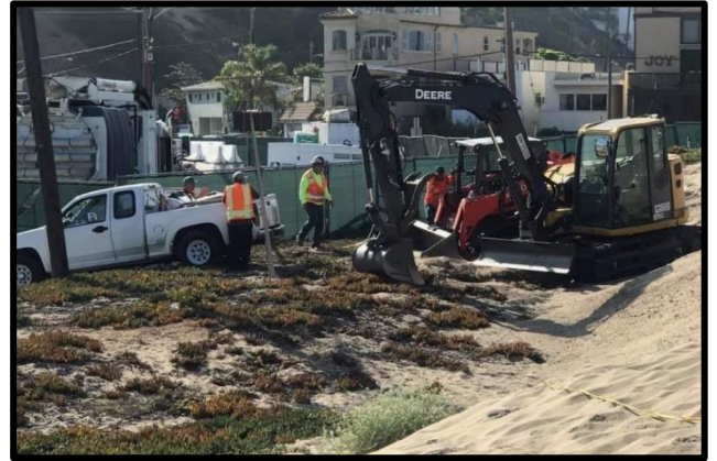
Unpermitted development, including the use of large construction equipment to grade coastal sand dunes and ESHA
